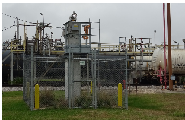
An OPSIS fence-line system installation.
